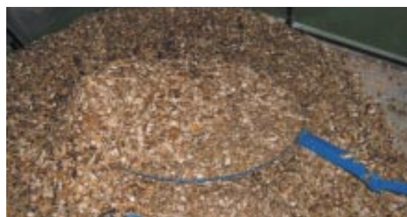
Inside the boiler feed system. Image: Marches Wood Energy Network
